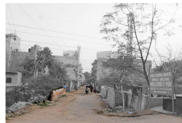
Under developed and ill maintained streets.
