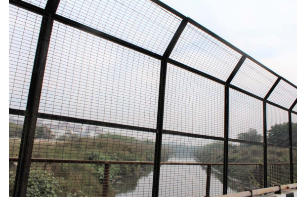
Prevailing unhealthy living conditions because of the open drain. Polluting the air, water and soil nearby.
