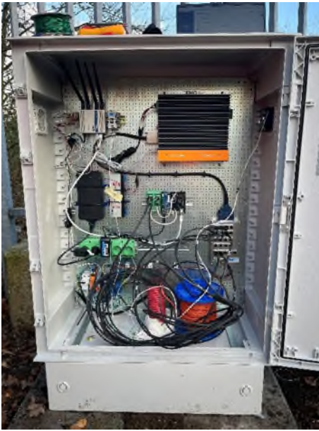
Figure 4. Photo of the equipment cabinet on the fenced terrain.
