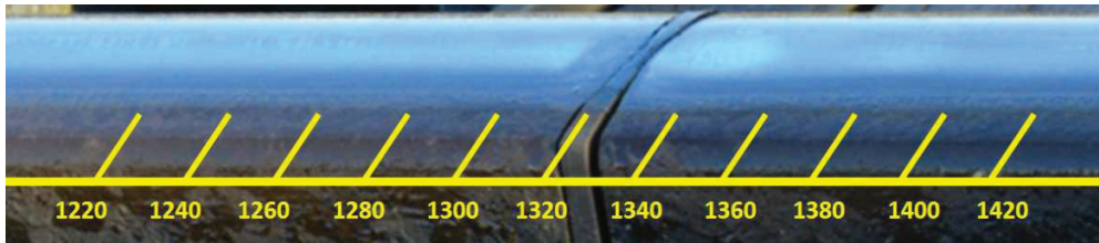
(b) In situ condition of the running band around the target IRJ
