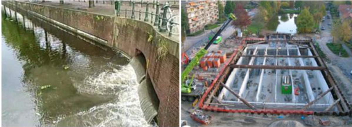
Figure 3.4 Combined sewer overflow (left) and construction of a CSO settling tank.
