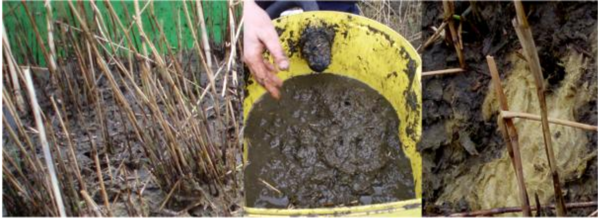
Figure 5.13 Accumulation of sludge at the surface of the filter bed.
