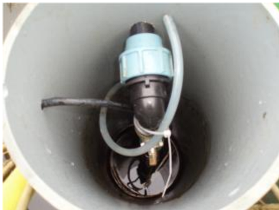
Figure 5.21 View inside the pump house: Available space for an adsorbent column.
