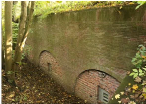
FIG. 4.55 Bunnik (NL), Fort bij Vechten. Solution to close the access to buildings while letting the transit of bats (design: BunkerQ) (F. Marulo 2020)
