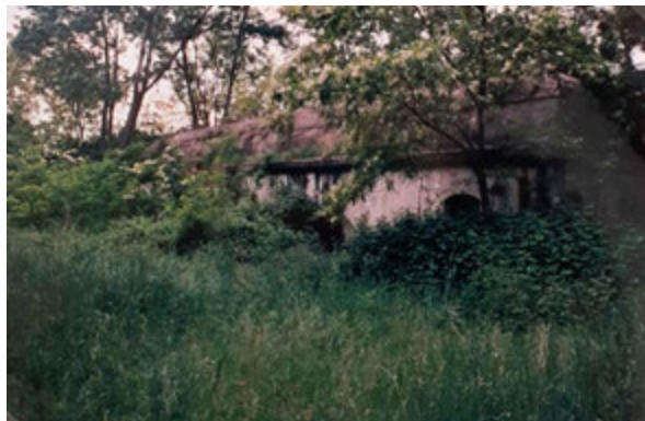
FIG. 5.19 Venice (IT), Forte Bazzera: the state of the fort after the abandonment of the military (1996) (ACCTM, Fond 1, Box Forti di Terra , File Forte Bazzera )
