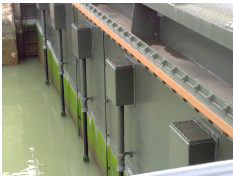
Figure 13. Door with five valves (underwater)
