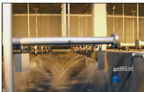
Figure 8 Spraying on top of a trickling filter
