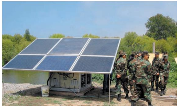
TRUNZ SOLAR DRIVEN WATER REVERSE OSMOSIS SYSTEM WITH BACK UP BATTERIES INSTALLED IN CHILE
