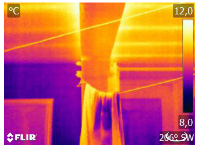
Figure 28: Infrared image of the back house. Own picture.
