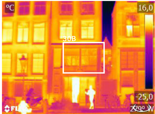
Figure 30: Infrared image of the exterior. Own picture.
