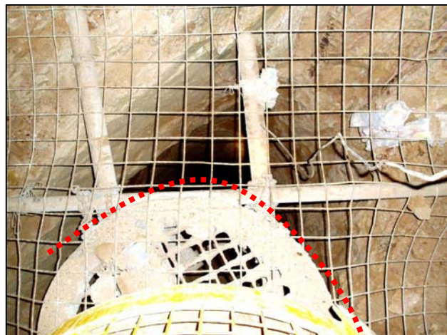
Figure 9 - Looking down what was intended as a round ventilation shaft. Overbreak has occurred along two intersecting fracture planes.
