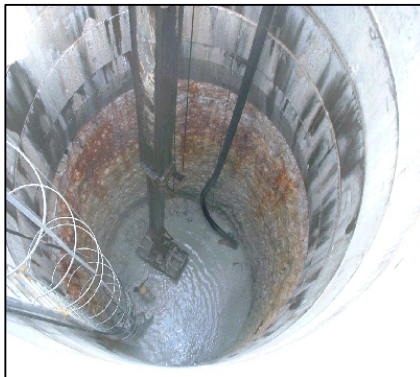
Figure 22 - Boom type excavator used to build a tunnel entry shaft in Abu-Dhabi
