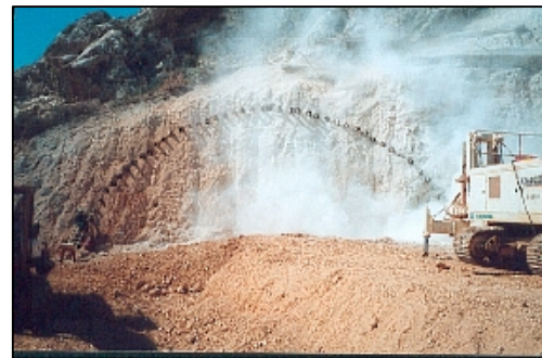
Figure 16 – Tunnelling example of forepoling in fractured rock in Greece [courtesy of the Geogineer Website, D. Zekkos]
