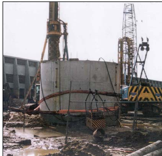
Figure 24 - Jack-down lining performed by Marin through soft clays. Pipes used for lubrication and grouting can be seen running along the outside of the lining
