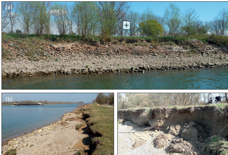
Figure 5.12. Unprotected upper banks in the Rhine River. (a) Test section near Worms on 12/04/2016, after riprap removal in 2011. (b-c) Section between groynes near Steinmauern on 23/03/2019, after protection removal in 2013 (courtesy of Petra Fleischer).
