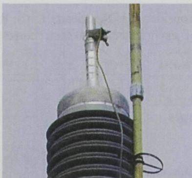
Figure 5.5: Close-up of the connection to the top of the termination used to inject artificial pulses.
