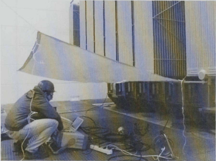
Performing partial discharge measurements in the radio frequency range, on an on-line transformer, under rainy conditions.
