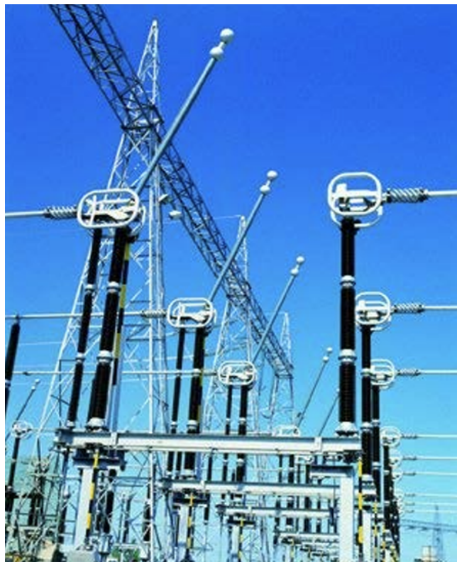
Figure 2.2: Example of an Air-Break Disconnecter Switch, from HAPAM B.V., as cited by [9]
