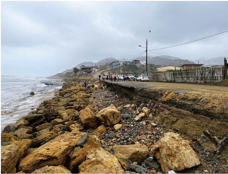
Figure 1.2: Coastal erosion becomes a direct societal hazard on developed coastlines. This photo from Ecuador, shows how coastal erosion may undermine coastal infrastructure and threaten coastal developments. While erosion is a natural process, it transforms into a coastal hazard where it threatens something of value. Photo: Arjen Luijendijk.
