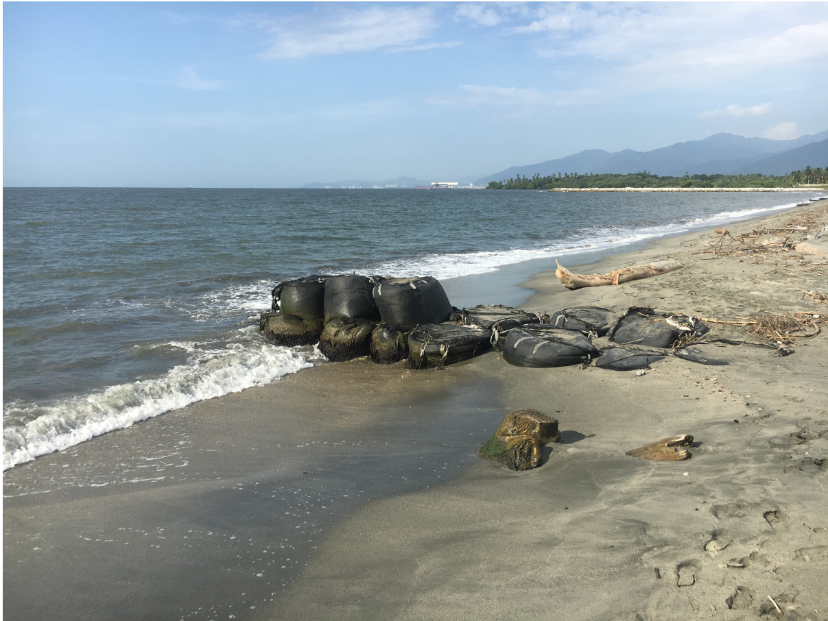
Figure 5.10: Groyne made out of sandbags at the Ciénaga coast
