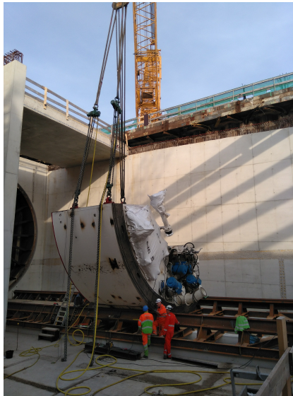
Figure AE.1: Starting structure of TBM in the starting shaft (Location: Rotterdamsebaan The Hague)
