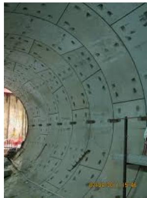
Figure 3.3: Concrete lining [15]. A close look give visual to the gaps in the lining where bolts can be installed. These bolts are placed to connect the individual segments to each other
