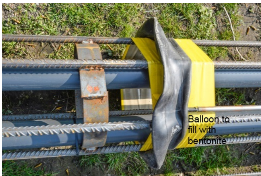
FIGURE C.2: Procedure for installing a neck. The picture shows the tire that can be inflated with bentonite. Picture provided by Deltares.
