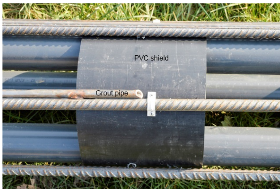
FIGURE C.1: Procedure for installing a bulge. The picture shows a part of the reinforcement cage where the end of a pipe is placed through which grout can be pumped. Picture provided by Deltares.
