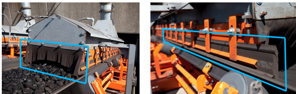
Figure 2.10: Rubber chute entrance curtains (left) and skirtboards (right) [1]
