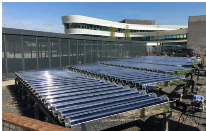
Figure 6: Virtu® PV/T-panels connected to the ATES system serving the office building in the rear; © Naked Energy, Christophe Williams
