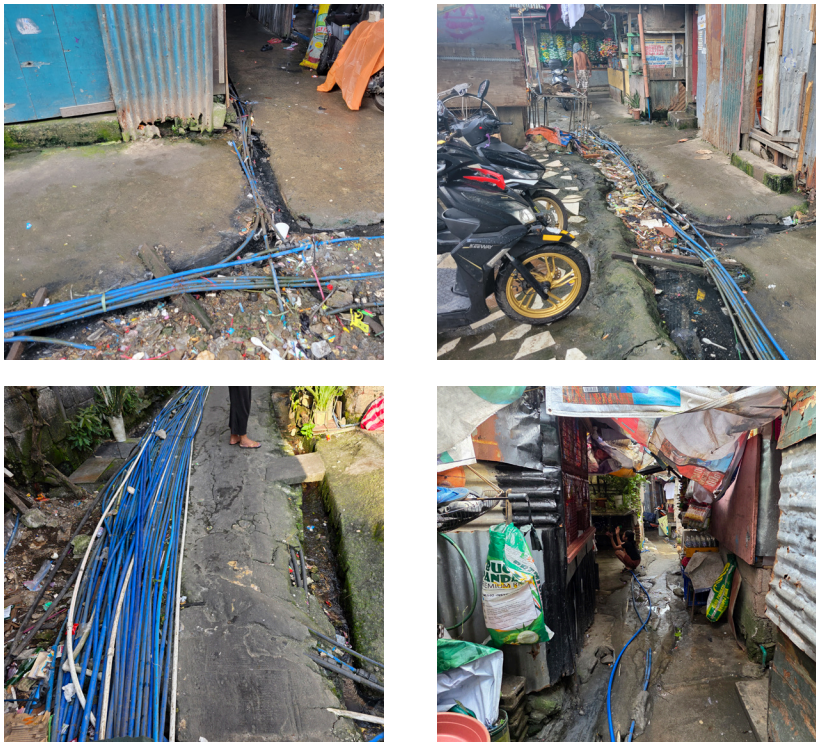
Figure 3.42 Concrete ground, exposed water line, and garbage
