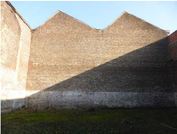
Industrial shed located on the Quai de l'Industrie 83b. Currently not in use, no visible windows or doors. (Image from Pierre Renard - Kaderstudio)
