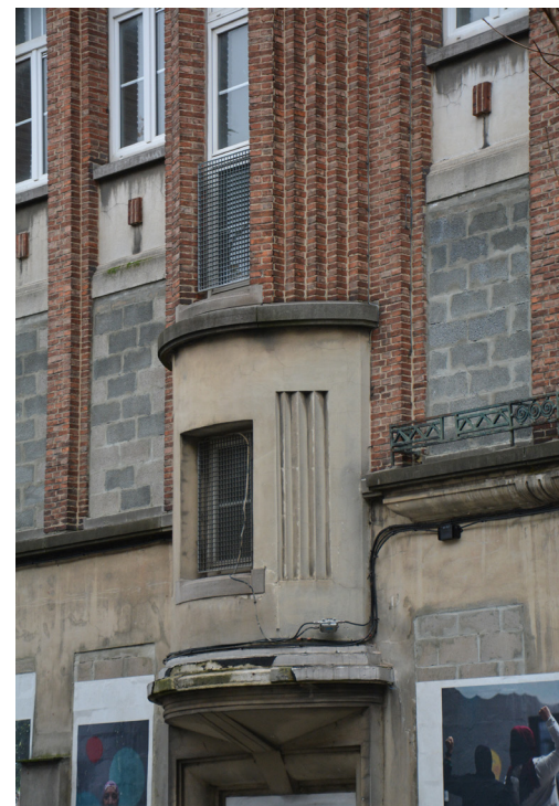
The building photographed in 2025/11/20. Serious decay and unused spaces are visible.
