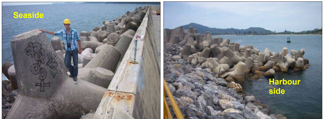
Figure 2-16 Left: The partly restored seaside protection. Right: The new and displaced Tetrapods at the head.
