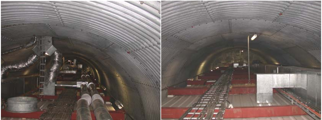
FIGURE 51: West tube, profile of free space in northern direction (left) and southern direction (right) (photograph: M. Wölk)
