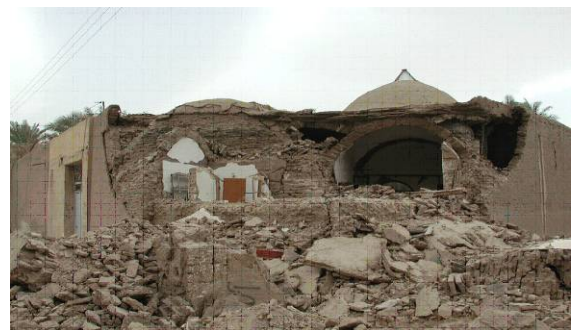
f) Parapet collapse on adobe building– 2003 Bam, Iran earthquake
