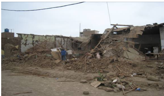
e) Roof collapse on adobe building – 2007 Pisco, Peru earthquake
