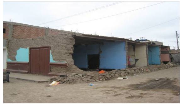
b) Out-of-plane wall collapse - 2007 Pisco, Peru earthquake
