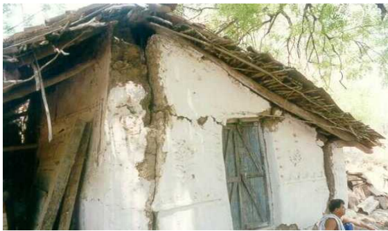
a) Vertical cracking and separation of walls – 1997 Jabalpur, India earthquake
