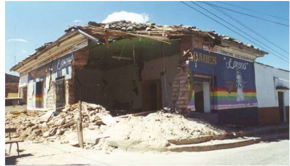
d) Total collapse of adobe walls – 2001 El Salvador earthquake
