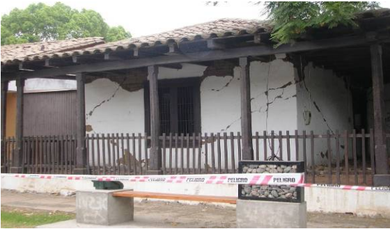
c) Diagonal cracking of adobe walls– 2010 El Maule, Chile earthquake
