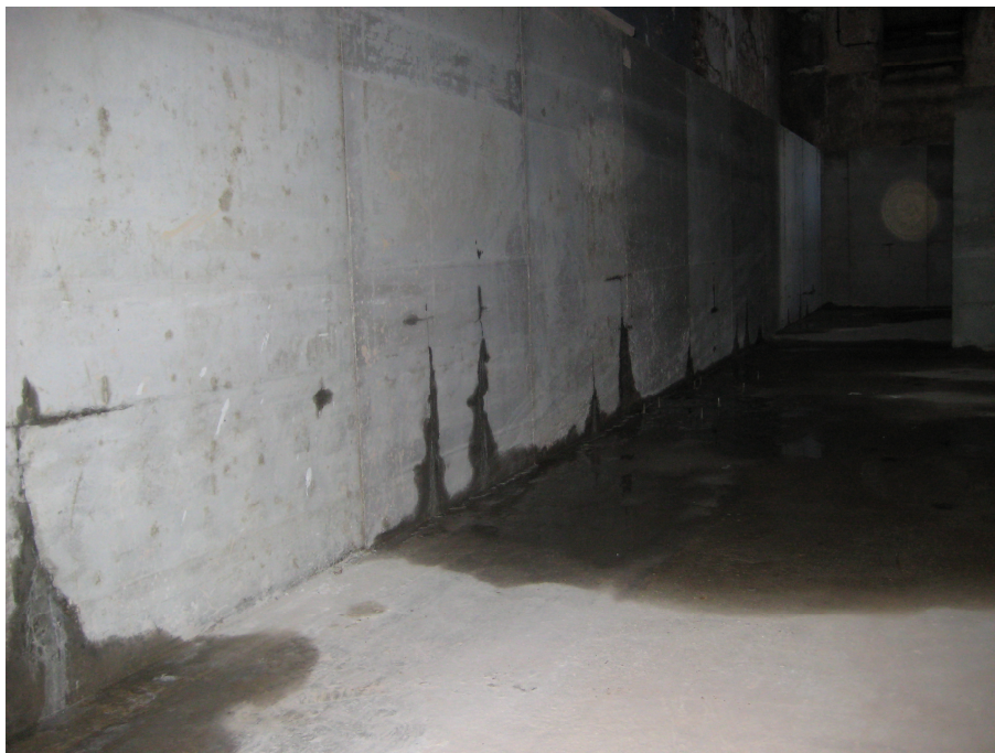
Figure 1.1 Example of water leakage of a cracked concrete wall casted on an existing concrete slab
