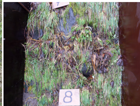
(b) Local damage after final overflow test ( t = 12:00 h, q_{max} = 165 l/m/s)
