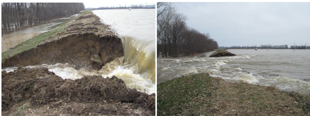
(a) Breached levee near the Mississippi river (2011)
