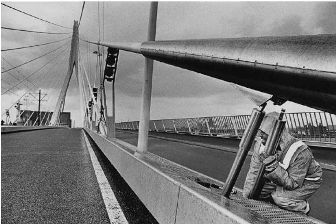
Figure I.1: Attachment of dampers at the Erasmus bridge to suppress rain-wind-induced-vibrations.
