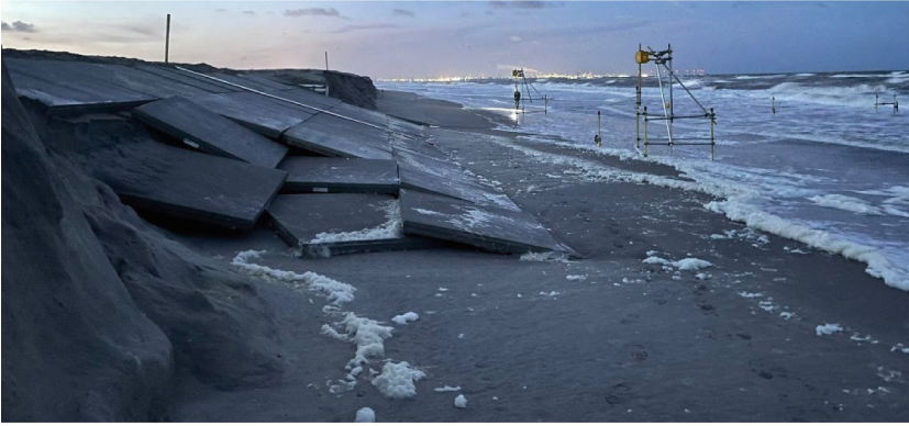
Fig. 5. The setup on 20 Dec 2024, after the first storm. The tiles start to collapse at the edges of the dike section. The container (background) is still fronted by a meter of sand.
