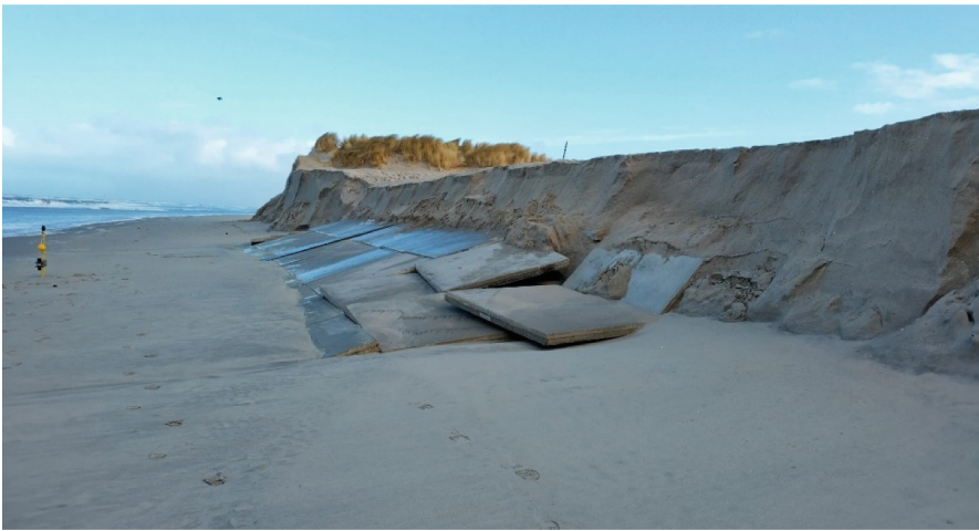
Fig. 6. The revetment of the dike-in-dune is partially uncovered after two storms. Erosion underneath the tiles causes the pates at the edges of the section to collapse.
