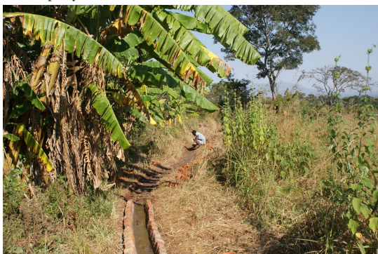
Figure A.51: Villagers start (under supervision of Resilience BV) with concrete lining of their irrigation canals to minimize leakage (June 2014)
