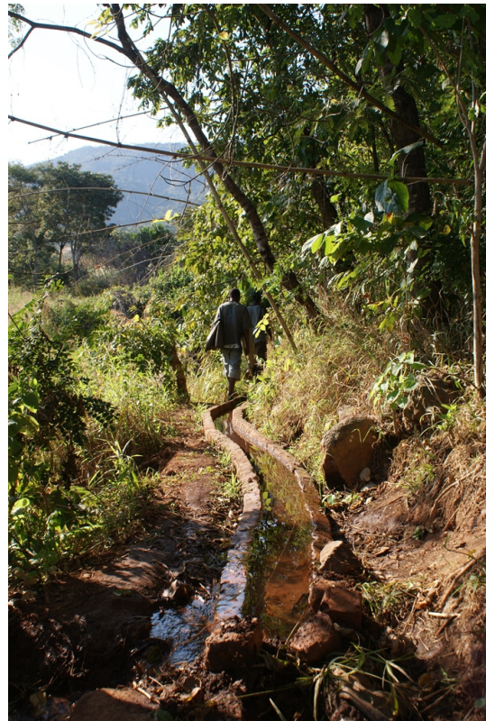
Figure A.52: Common practise in lined and unlined irrigation canals; leakage of water along the length. Most of the water already flows back to the original stream within the first meters (June 2014)
