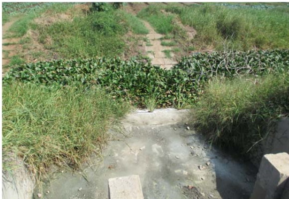
Figure 8.44 Facultative outlet 1 (empty)
