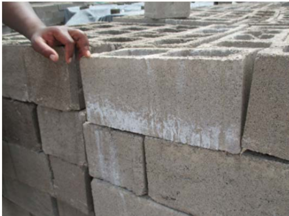
Figure 8.23 Evidence of efflorescence
