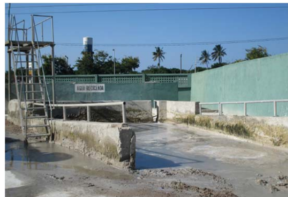
Figure 8.30 The entrance of water recycling system
