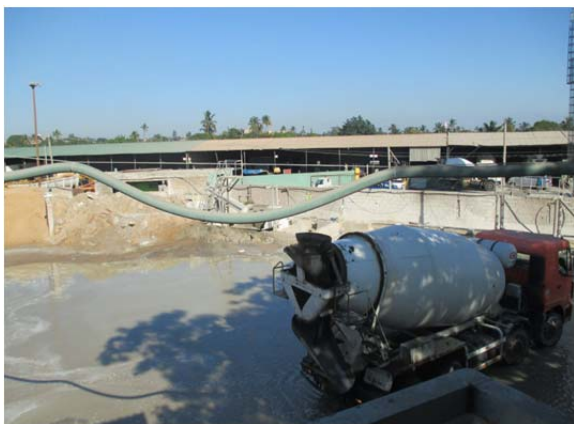
Figure 8.33 A truck having been washed and the used water collected in a pond
