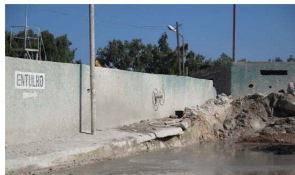
Figure 8.31 The disposal and sludge storage
