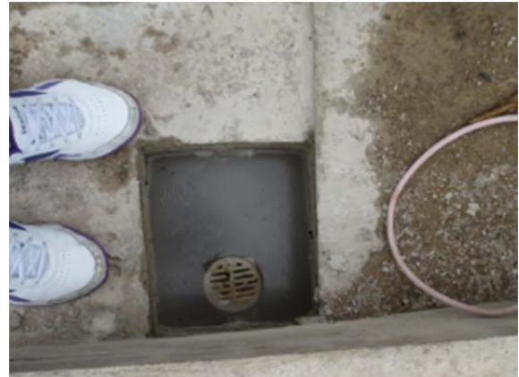
Figure 8.9 Drain connected with the decantation tank
