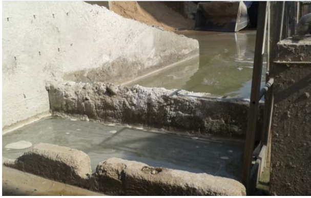
Figure 8.19 Open ditch that transports the collected wastewater (after being used for washing the trucks) into a decantation system
