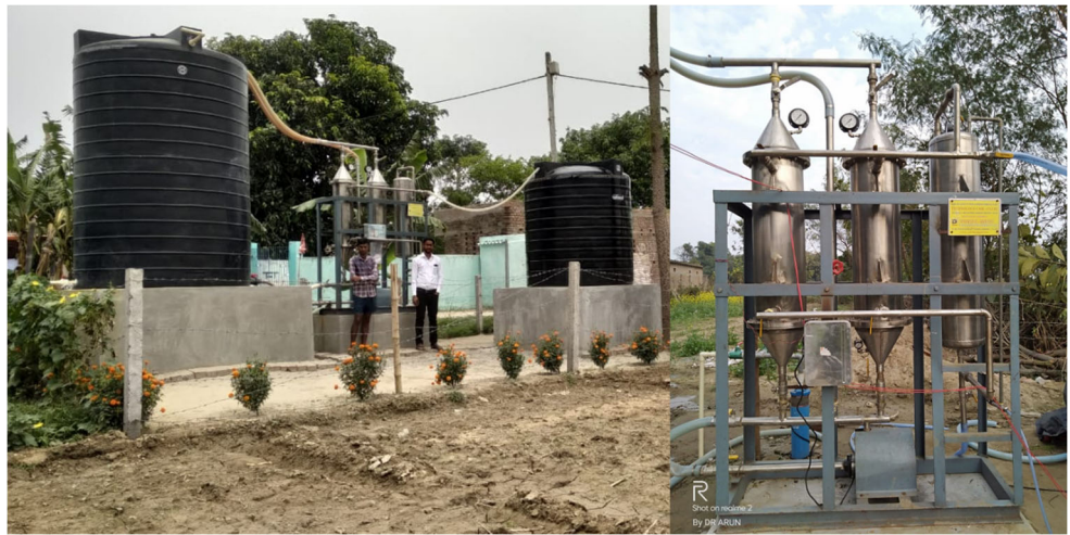
Fig. 9 Mitigation unit (arsenic filter) installed in the village
