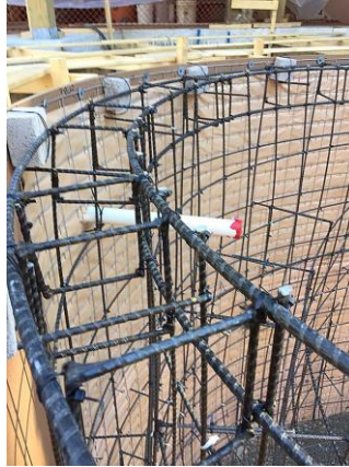
Figure 2.1.7: BFRP in swimming pool (Basalt.Guru, 2016)
