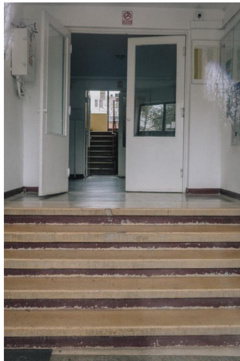
Figure 6: Nistor, Cristina. 2024. Flight of stairs leading to the elevator, no handrail. Photograph taken by the author.
