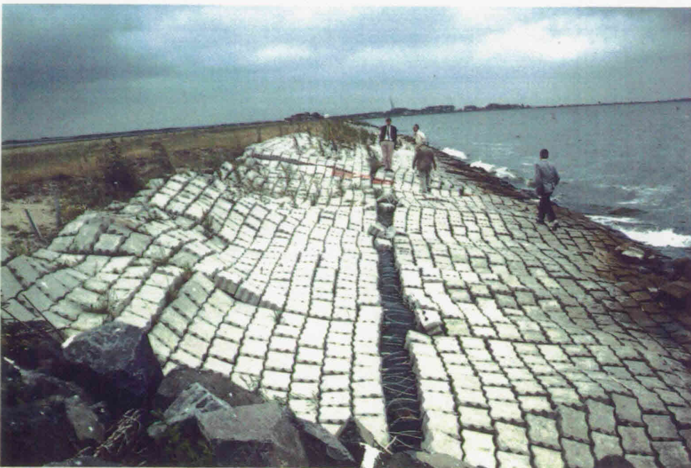
Picture 8 : Beto-mat; impression of the deformation of the slope. On the foreground the transition to the rip-rap reference section
