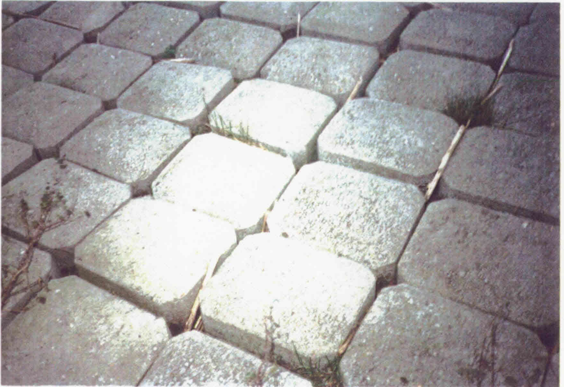
V.O.B.-mat, fixed to a geotextile and placed on minestone and on sand (Houtrib-dike)
