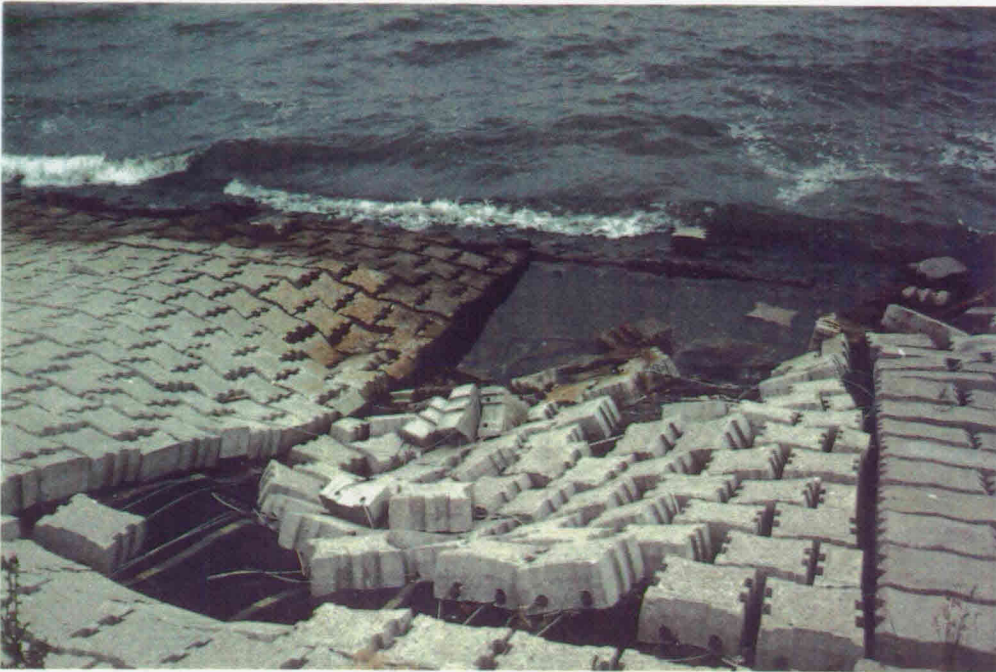
Picture 7 : Armorflex-mat; detail of damage close to the transition to the Beto-mat
