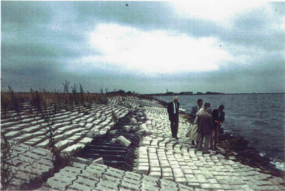
Picture 5 : ASAM-mat; part of the bank protection slid down along the slope. On the foreground, the transition to the Armorflex section
