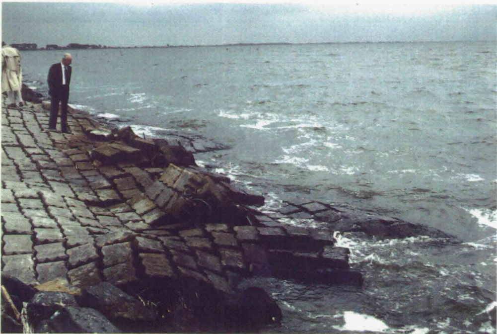
Picture 12: Beto-mat: part of mat slid down and pushed up against lower mat sections (detail of picture 11)
