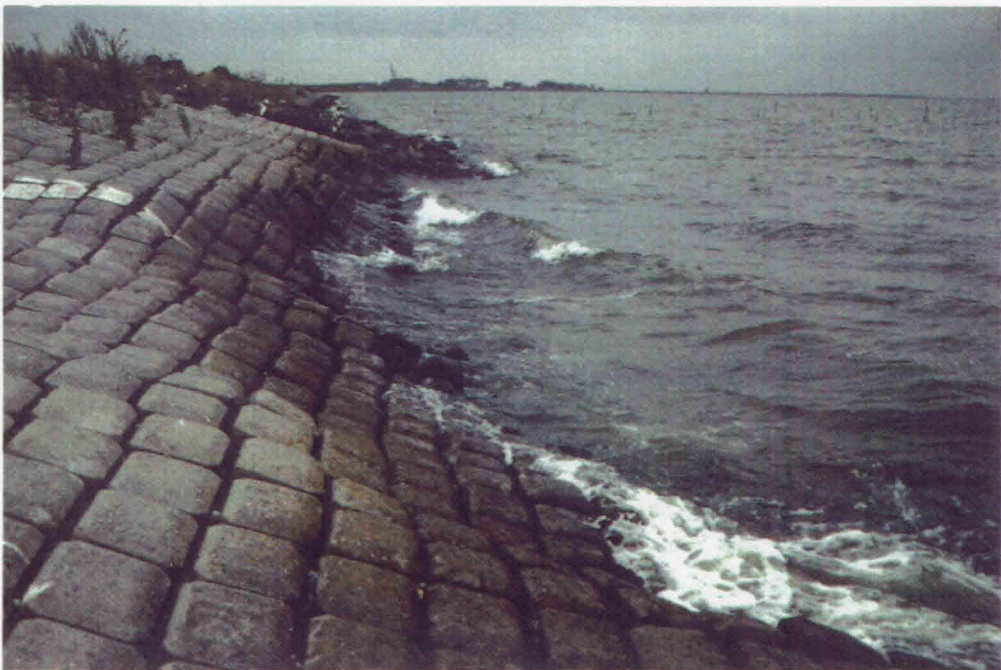
Picture 2 : V.O.B.-mat; detail of the slope deformation
