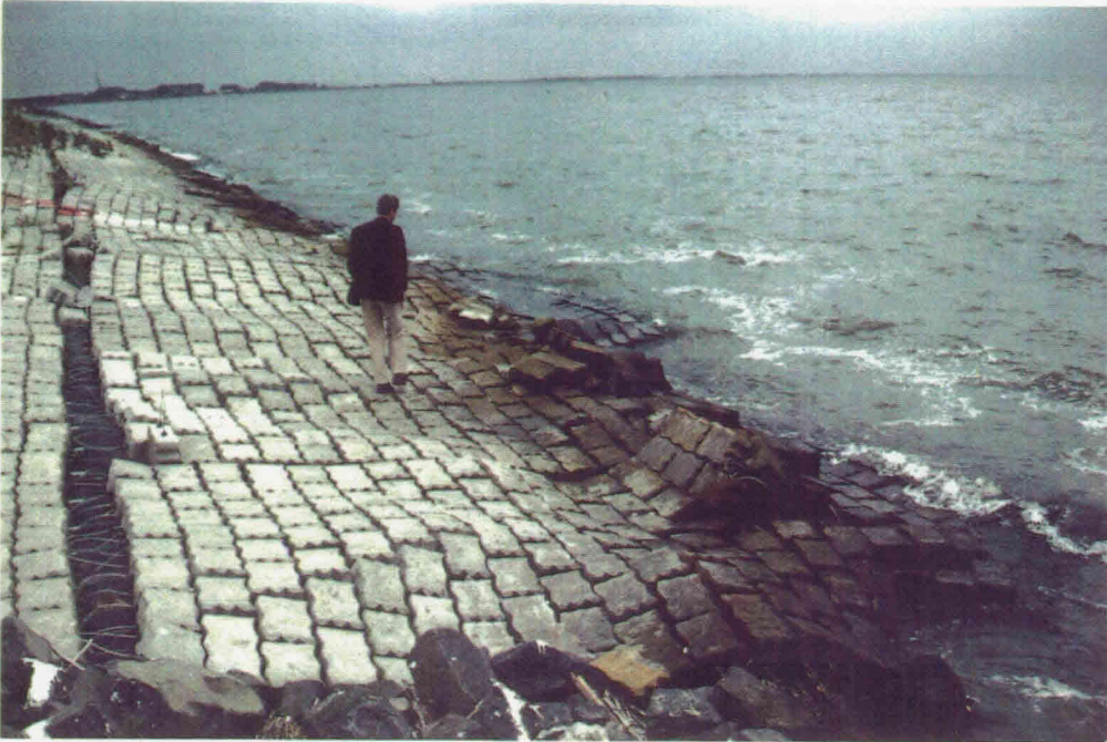
Picture 11: Beto-mat; over all picture of slope deformation and damage
