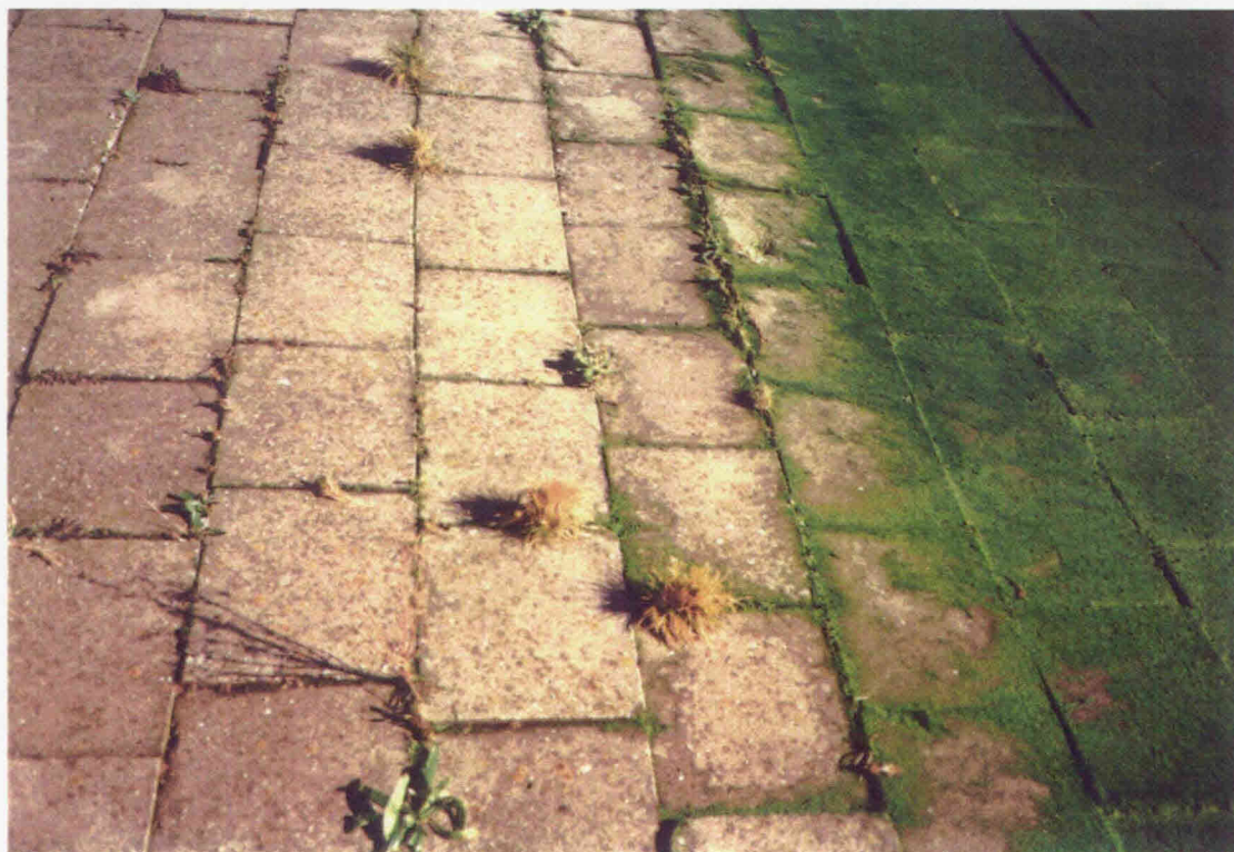
blocks placed on geotextile, clay, on gravel and on sand (Hartel Canal)
