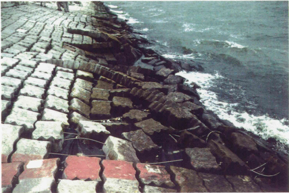
Picture 9 : Beto-mat; detail of damage
