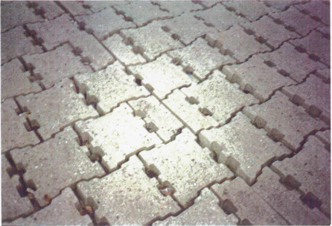
Armorflex-mat placed on a geotextile on minestone (Houtrib-dike), showing joint between 2 adjacent mat sections
