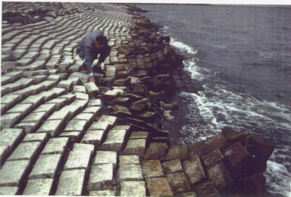
Picture 4 : ASAM-mat; detail of damage
