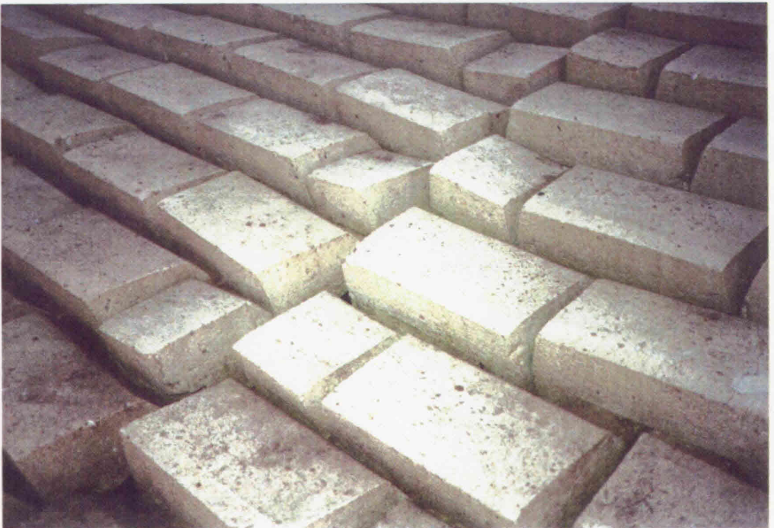
ASAM-mat, placed on a geotextile on minestone and on sand (Houtrib-dike), showing joint between 2 adjacent mat sections
