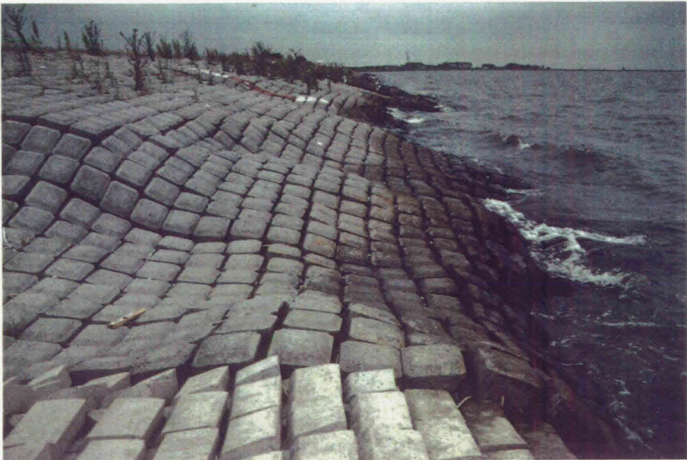
Picture 1 : V.O.B.-mat; impression of the deformation of the slope. On the foreground, the transition to the ASAM-mat
