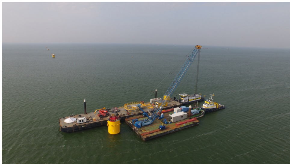
Figure I.6: Aerial photo of the shaker on the monopile (MP45) tested as part of the DISSTINCT project in the Westermeerwind wind farm. Source: Versteijlen et al., 2016a
