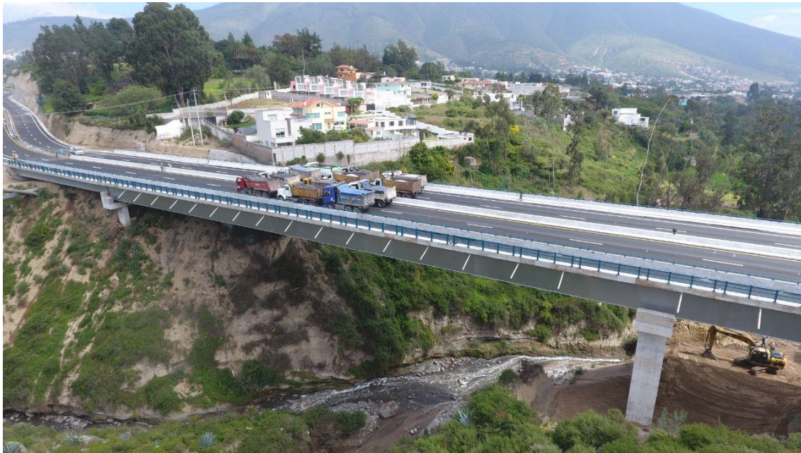
Figure 2. Load testing of a new bridge prior to opening with trucks – Villorita Bridge, Quito, Ecuador. Photograph by T.A. Sanchez. Used with permission.
