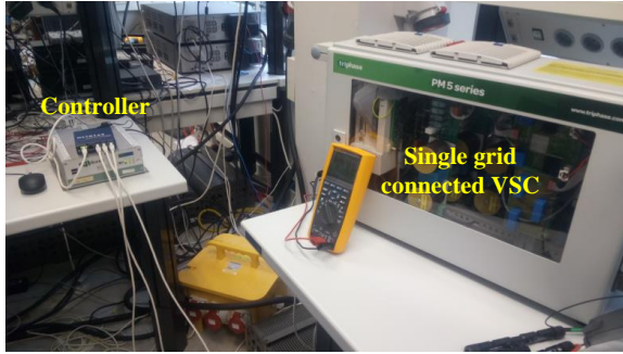
Figure 6.14: Two-level VSC Triphase/PM5F30C used for experimental validation.
