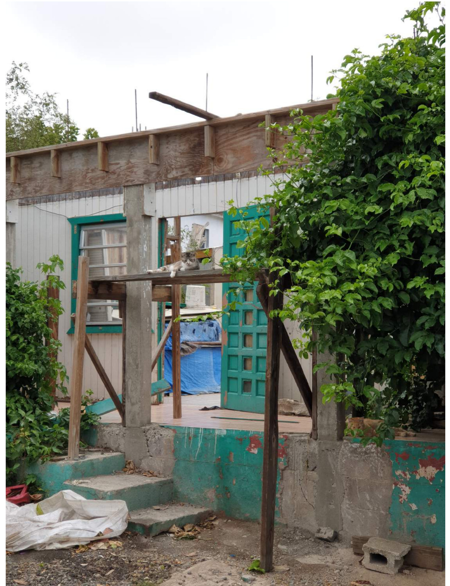
House damaged by hurricane Irma situated in Cole Bay next to local host Kim. Image by Danique Landburg
