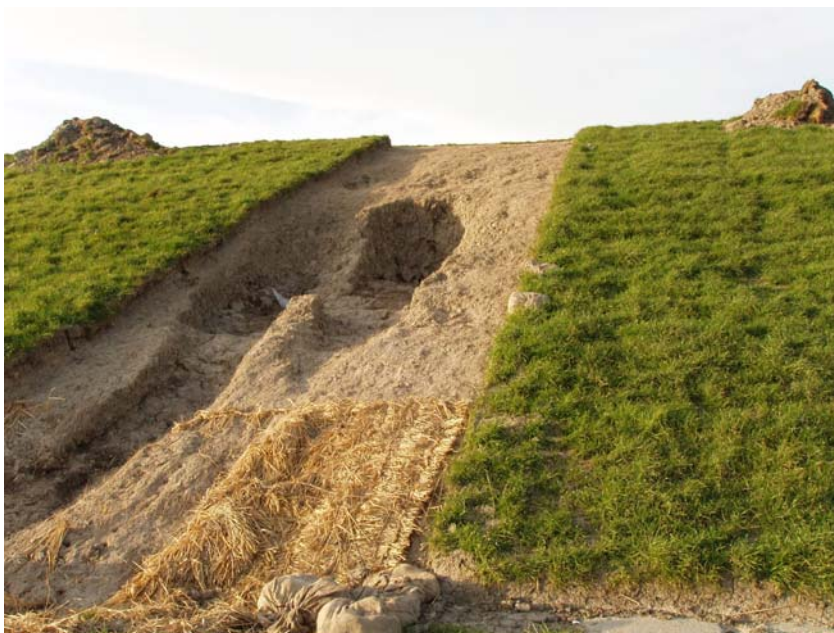
Figure 11-5: Deep scour holes after wave overtopping of 10 l/s/m
