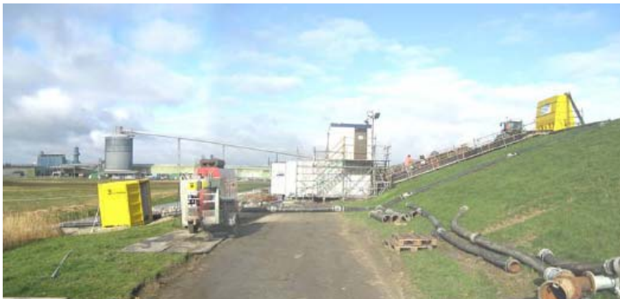
Figure 2-4: Overall impression of pumping system
