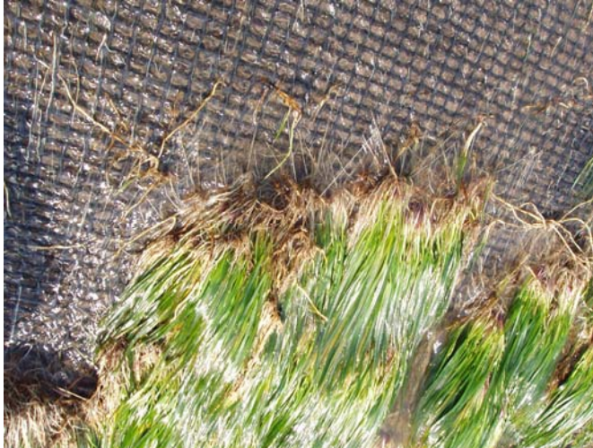
Figure 10-6: Anchoring of grass roots to the Geogrid near the artificially removed grass cover
