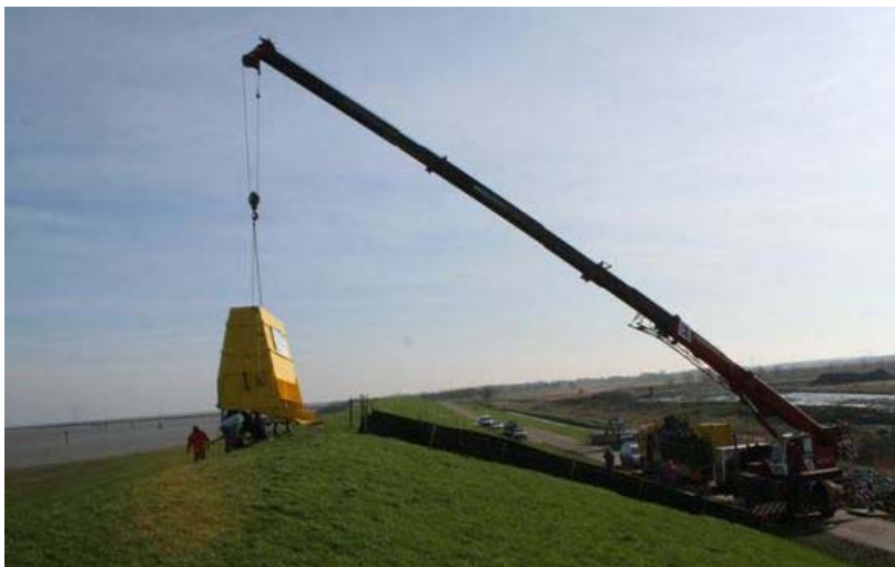
Figure 4-6: Placement of the simulator at the test site by a large crane
