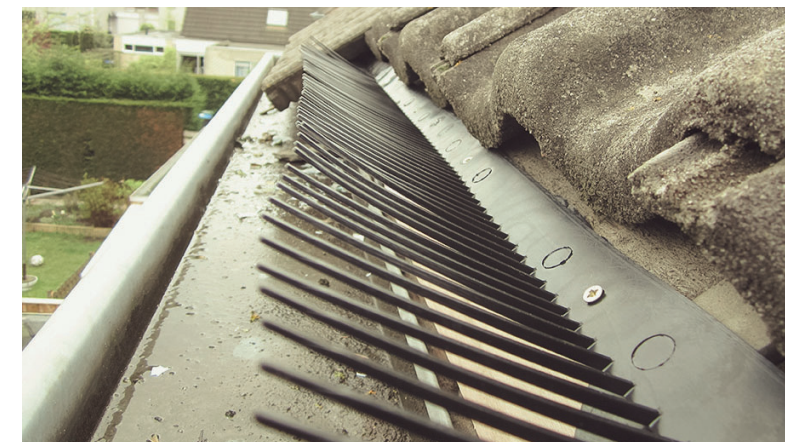
Figure 6. Bird scrap for keeping birds out under roof tiles. (Adapted from Traas building care, n.d.)
