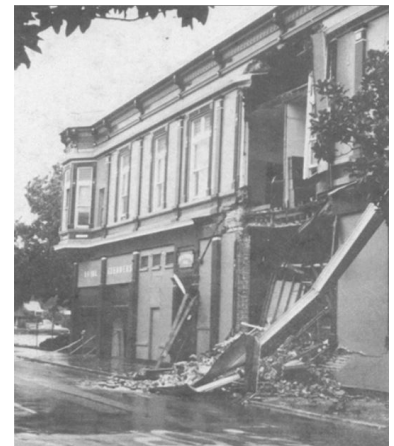
Figure 3.4: Out-of-plane failure over two levels due to flexible floor, (Bruneau, 1994).
