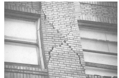
Figure 3.3: In-plane cracking of pier due to shear stresses, (Bruneau, 1994).
