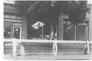
Figure 3.2: Failure of anchorage and slip of floor inside the building, (Bruneau, 1994).
