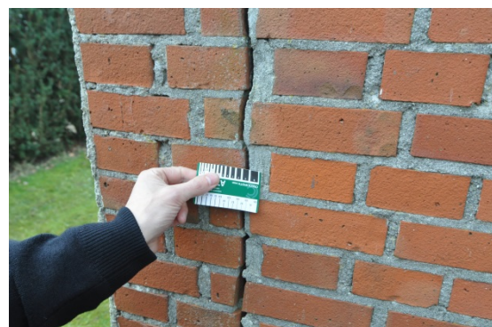
Figure 1: Damage inspection of masonry house in Groningen
