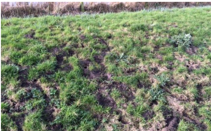
Figure 3: damage to levee as a result of a mice plague. Source: (Deltares, 2014)
