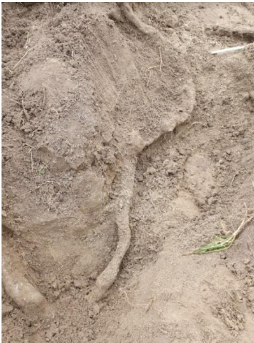
Figure B3: Tunnel leading towards burrow hole that showed grouted pouring out, labelled as 1 in Figure B1
