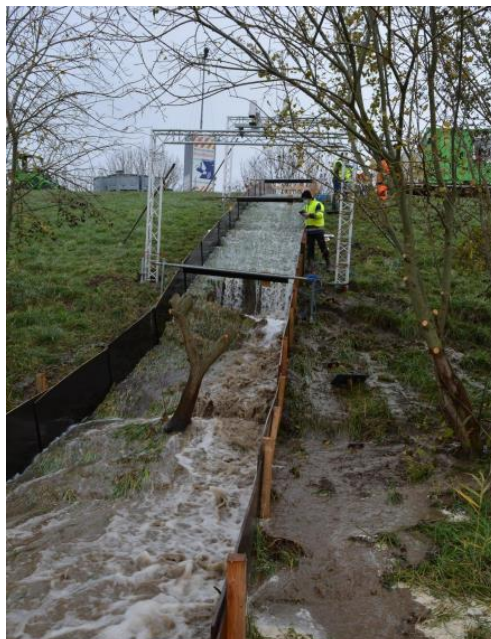
Figure 2: Erosion damage at experiment site as a result of mole burrows, source: (Koelewijn, Kieftenburg, & Hûsken, 2020)
