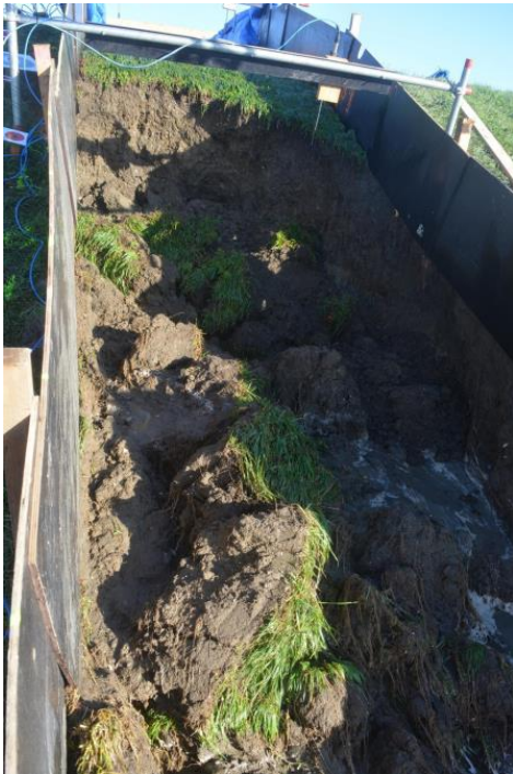
Figure 4: Damage due to reduced erosion resistance from fox burrows. Source: (Koelewijn, Kieftenburg, & Hûsken, 2020)
