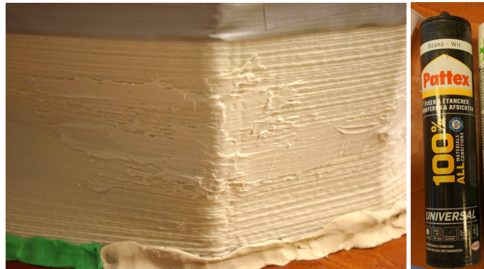
Figure 7.14: Filling the cracks. Left: surface of the mould after fixing the cracks. Right: the filler.
