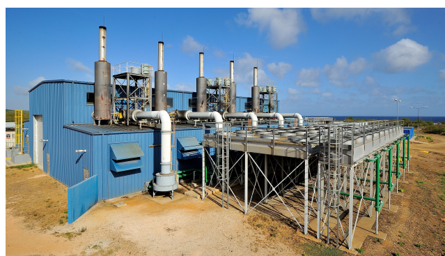
Figure 3.6: Diesel plant on Bonaire (Source: Contourglobal (2017))
