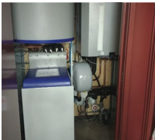
Figure 6 The installation room in a ZE house. It houses the equipment, but is a black box to residents.
