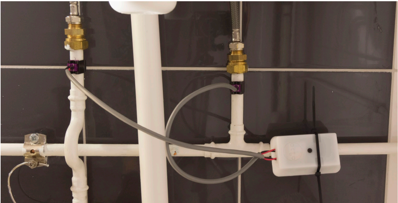
Figure 4. Installed stoppage sensor
