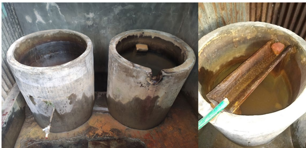
Figure S1: Pictures of sampled groundwater household-scale treatment plant in Manikganj. Left: missing aeration tray. Right: aeration tray present
