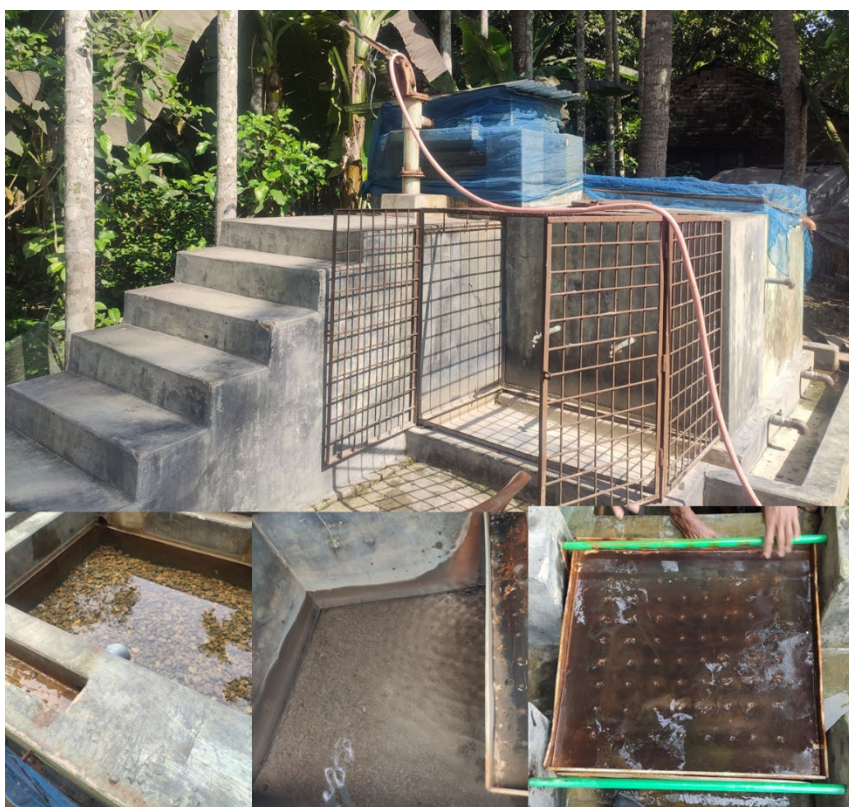
Figure S2: Pictures of sampled community-scale treatment plant in Satkhira. Top: overview picture of the whole plant. Bottom left: Filter 2 (stones), bottom middle: Filter 3 (sand), bottom right: aeration plate
