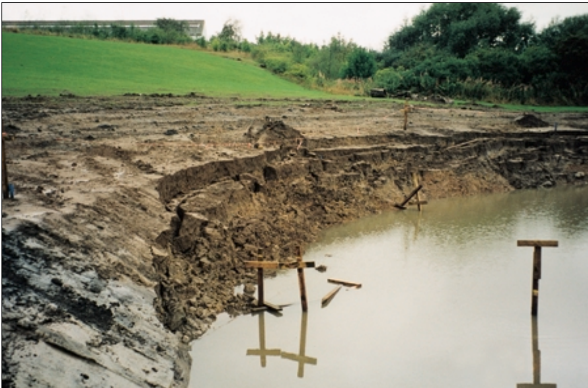
Slipped slope during work – September 1995
