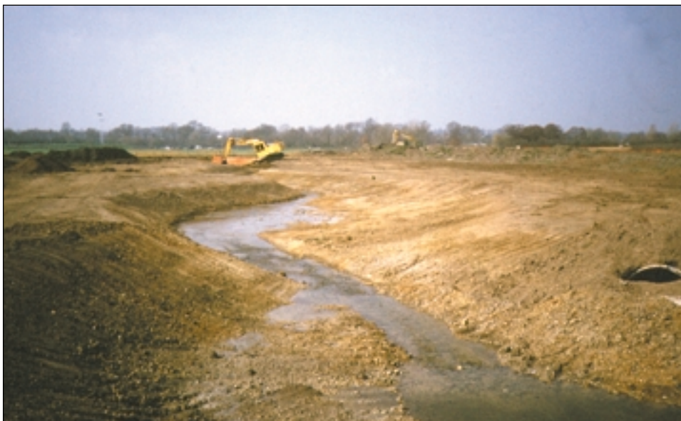
Looking downstream at the shallow bank slopes. The severed culvert still visible
