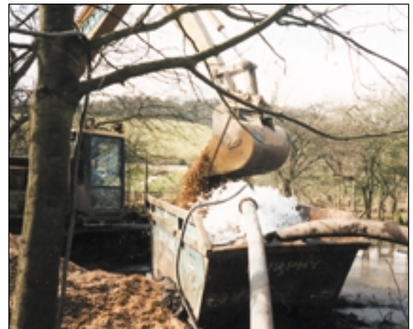
Pumping apparatus in operation
