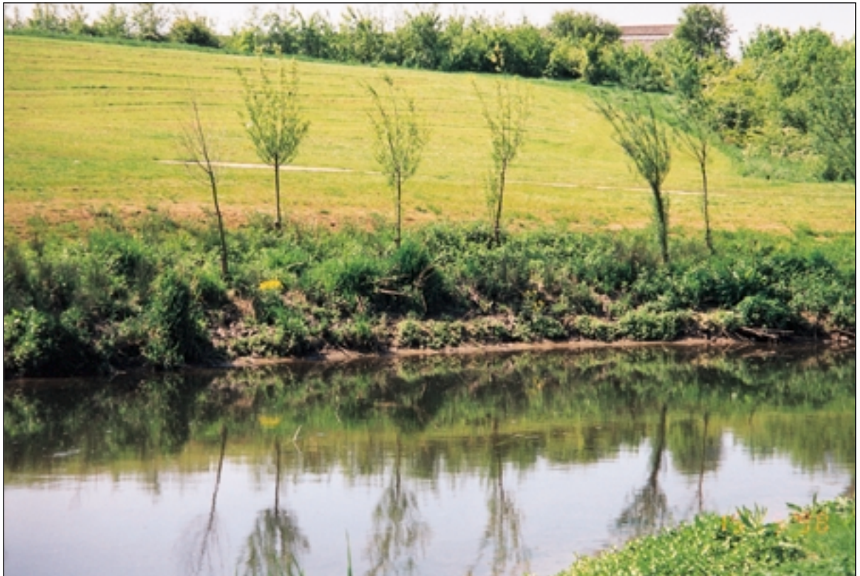
Slipped slope 2 years after repair – 1997
