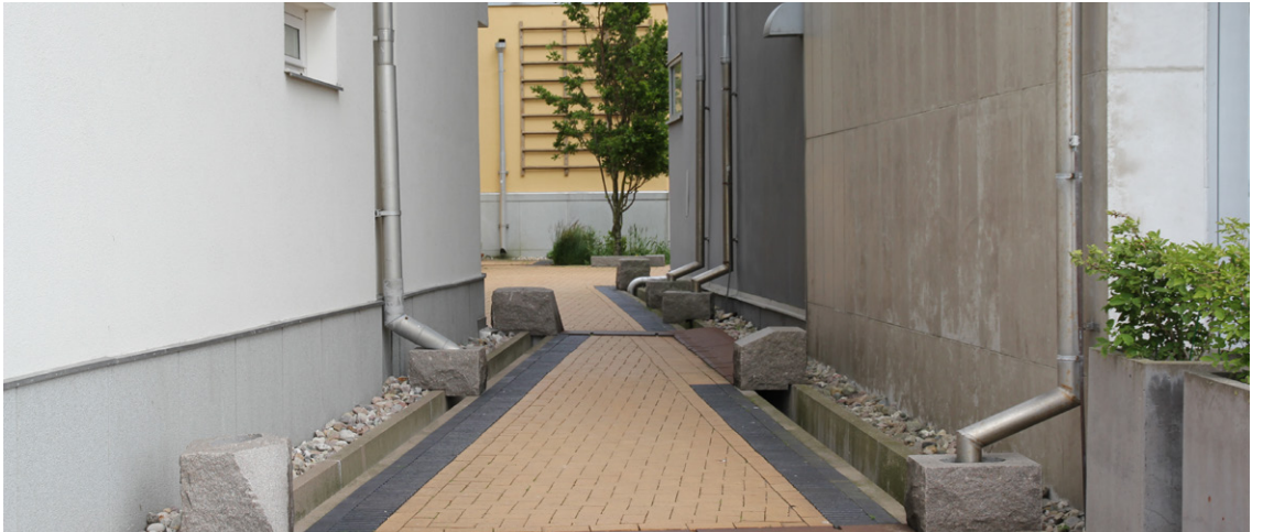
Figure X: Drainage canals with granite blocks, black concrete slabs and steel plates.
